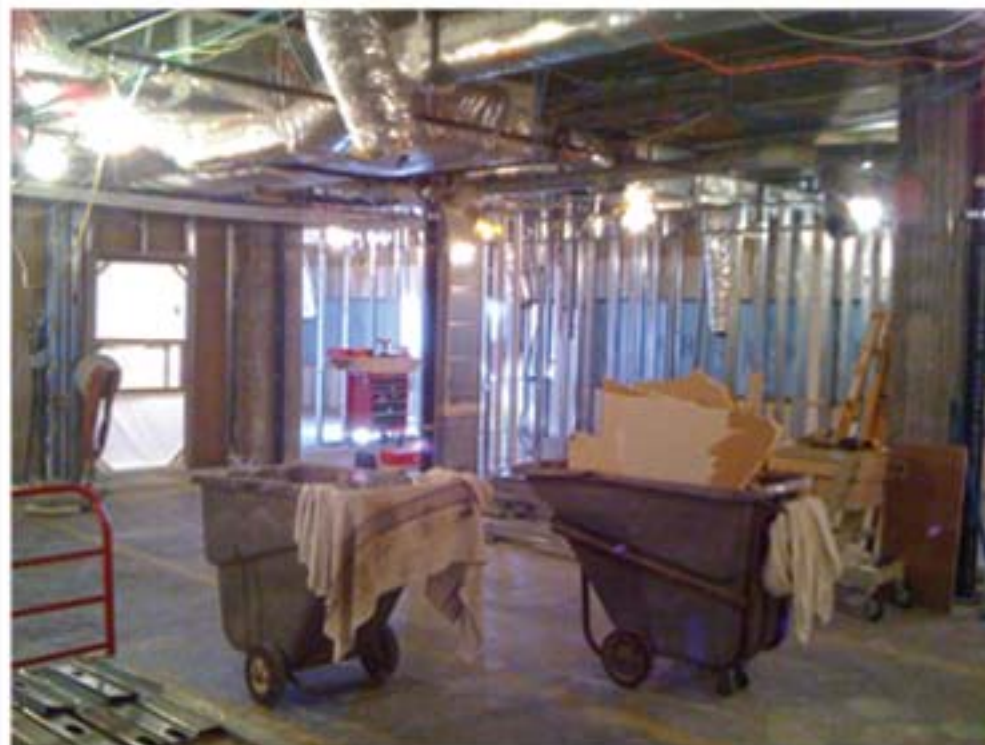
What used to be office and exam room space on the east side of the Heart & Lung Center has been torn down to pave the way for an expanded holding area for Cath Lab patients.
