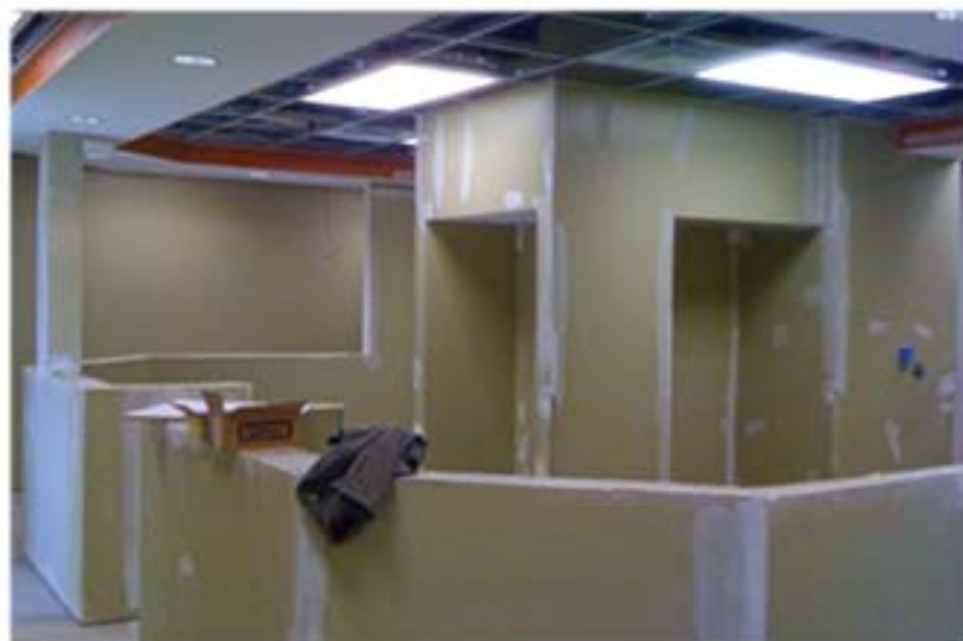
A work station just off the main lobby in the new cardiology building begins to take shape.
