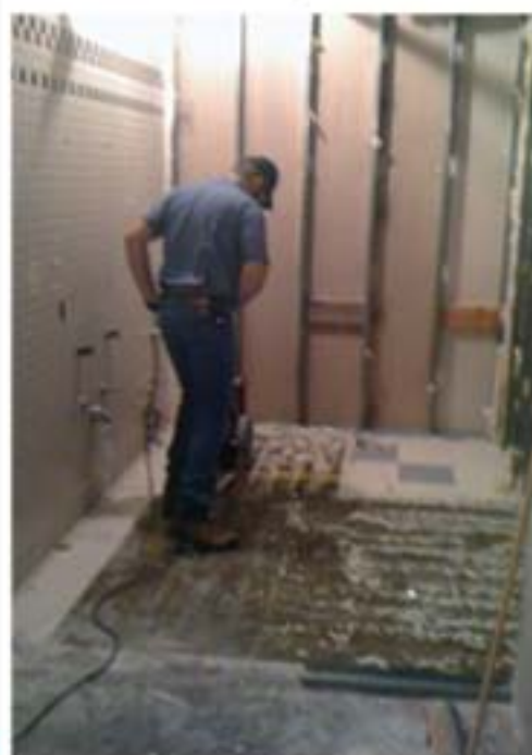
Cory Pullins of the JPMC Maintenance crew removes floor tile during the remodeling of the Heart & Lung Center on the eighth floor of the Patient Tower.
